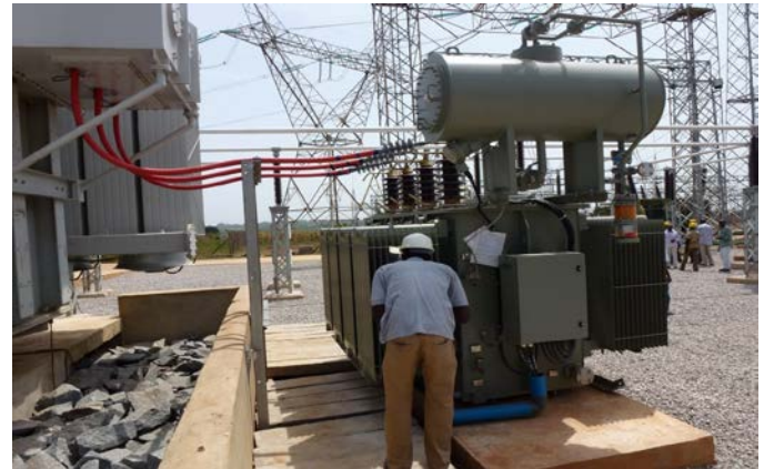
A 132/33kV SS Undergoing Pre-commissioning Test/Checks
