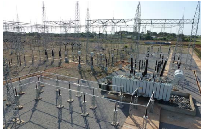
132/33kV Mando SS Commissioned
