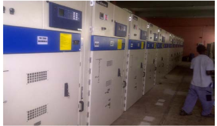
132/33kV Control Panels
