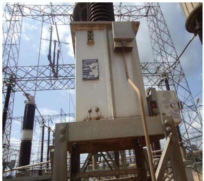
A Circuit Breaker at a Substation
