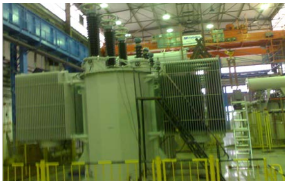
60mva, 132/34.5kv power transformer for Obudu substation
