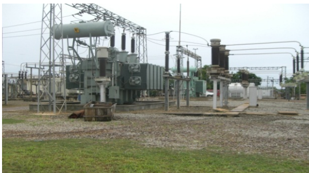
Abakaliki S S showing area for extension works for Ikom 132kV TL bays/equipment
