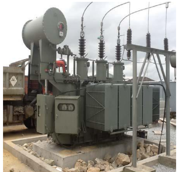
A 7.5 MVA Transformer on Plinth
