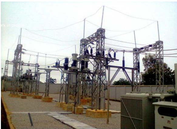
Pankshin Injection Substation
