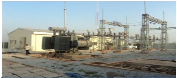
1x7.5MVA Kaduna Industrial S/S
