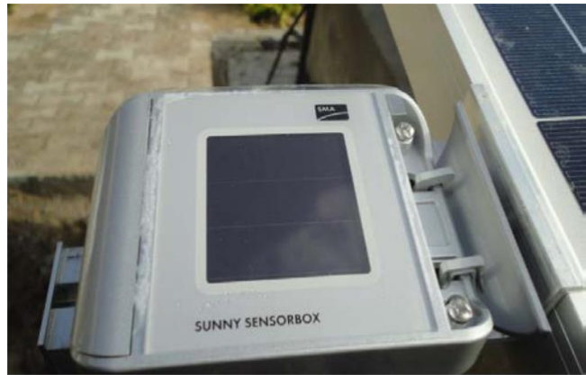
Sunny Sensorbox, part of the Solar PV System
