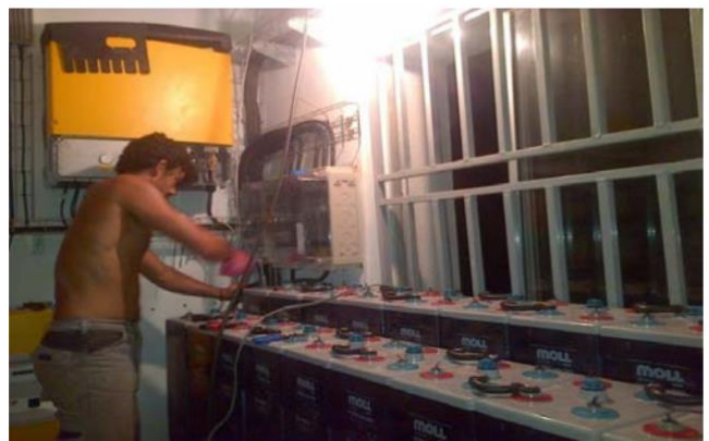
Connection of the solar batteries to the inverter in the control room.
