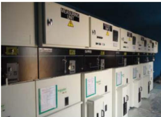
Control Room of the Wind Farm
