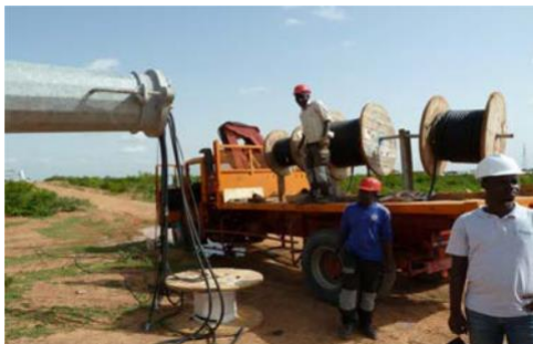
Low voltage connections
