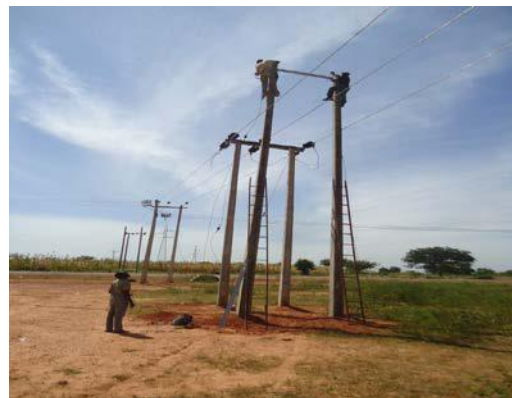
33/11kV line route from the Windfarm to Katsina substation
