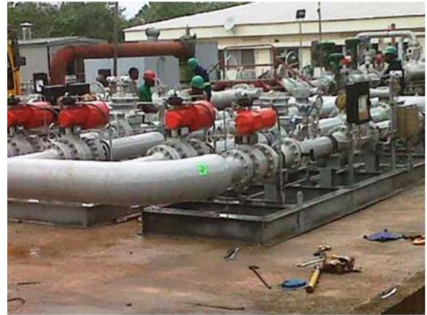
Omotosho: New NDPHC Power Plant four-stream Metering Facility mounted on two skids capable of delivering 280mmscf/d
