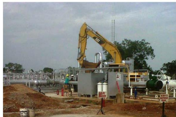
Geregú: An excavator preparing the pipeline approach to the gas sales manifold of the new NDPHC metering facility
