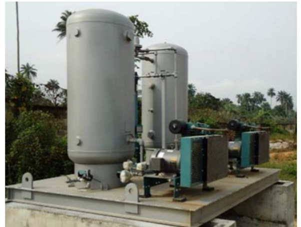
Calabar: Air Compressor on Foundation
