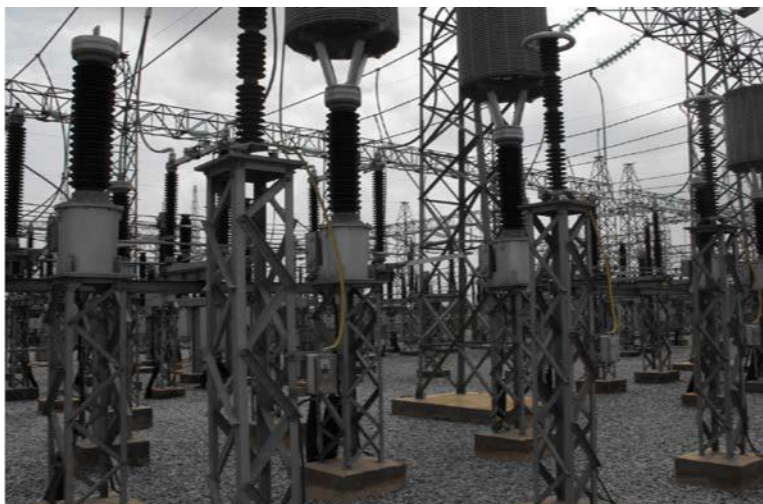
Wavetraps at a Transmission Substation
