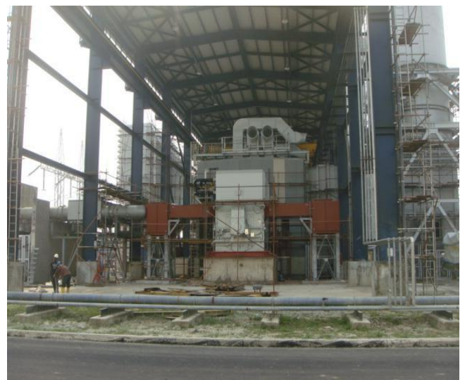
Gas Turbine Hall in Calabar
