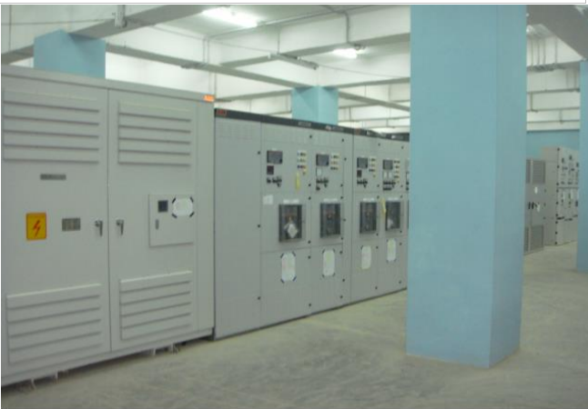
Central Control Building CCB at Calabar Power Station
