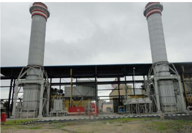
Back View of GT3 and GT4, Sapele Power Station
