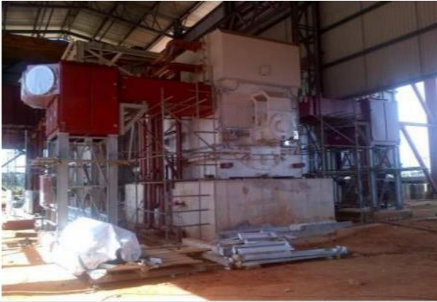
Generator and GNAC at Egbema Power Station
