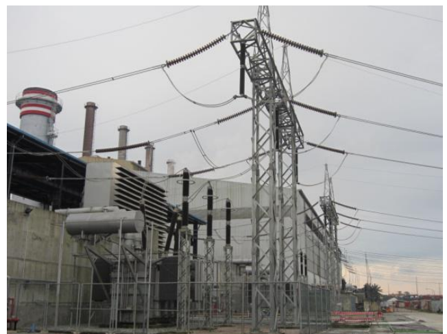
GT 1 with transformers connections at Sapele
