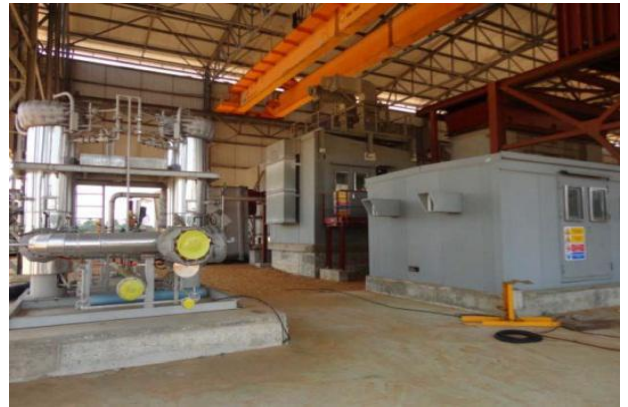
GT Ancillary Equipment at Omoku
