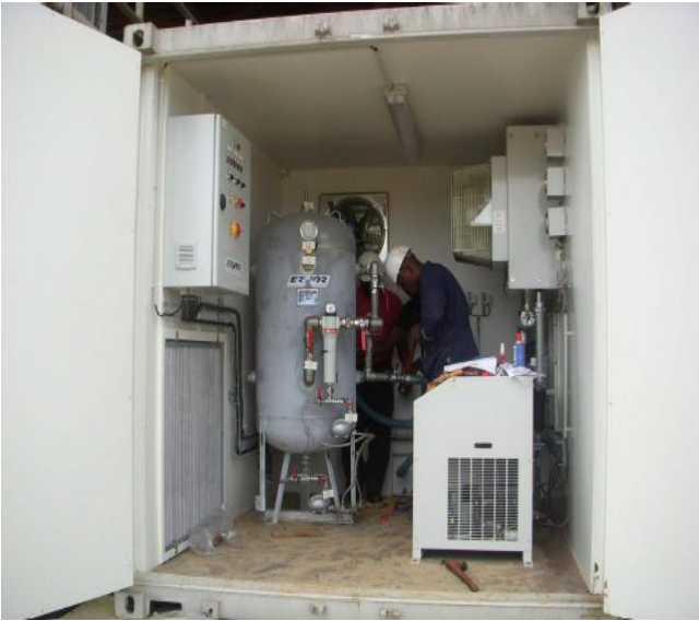
Air processing unit for GT 2 at Gbarain
