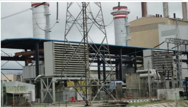
Front view:-GT 1 and GT 2, Sapele Power Station
