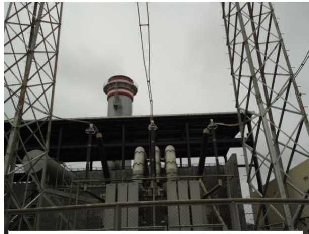
Generator Step Up Transformer (GSUT) at Egbema
