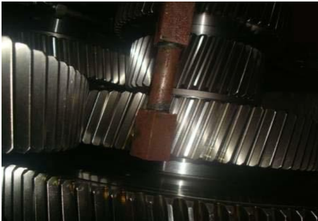
Rust on Spray Pipe - Discovered during boroscope Inspection
