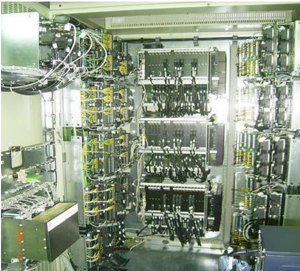
Mark 6 Turbine Control Compartment
