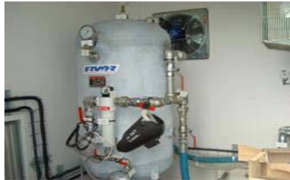
Air Processing Unit (APU) System
